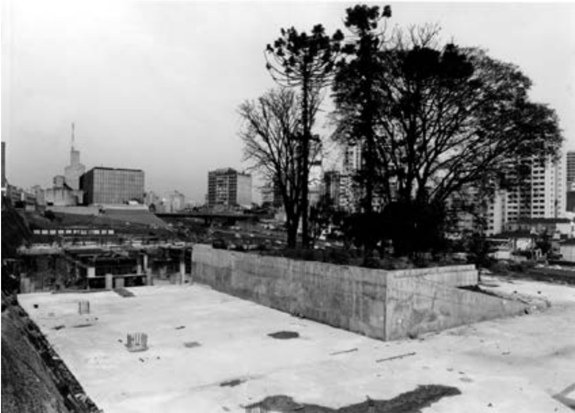
Centro Cultural São Paulo under construction. The photo shows the grove that was created in the middle of the work. This grove was original to the land. Photo: Waldemir Gomes de Lima
